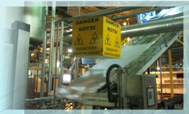
Figure 2: Nucleonic gauge in use with the signage displaying radioactive source and emergency contact details
